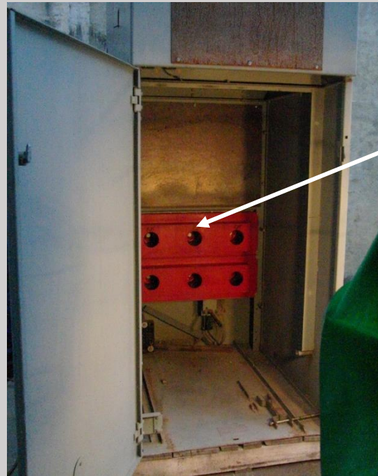
Rack-in Style Switchgear Cubicle - Shutter Removed
