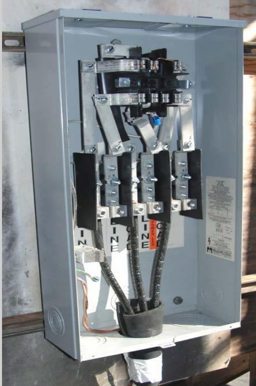
BYPASS METER SOCKET
